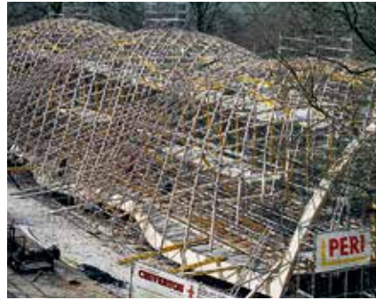
MULTIPROP Props carried the timber construction and facilitated the curved shape of the gridshell.
