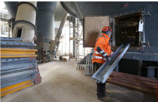
The lightweight, easy-to-handle PERI UP components were fed easily into the facility through small openings and then brought into position.
