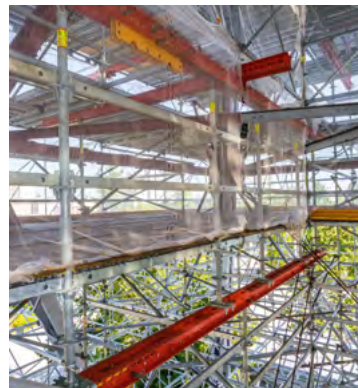
The PERI scaffolding solution for scaffolding the complex truss construction was based on PERI UP and VARIOKIT – two systems combined with each other.
