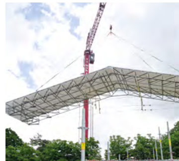
Pre-assembly of the truss units is carried out from a safe position on the ground. Lifting is done by crane.
