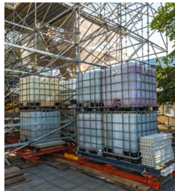
Well combined: VARIOKIT system components were used to distribute the load from the offset verticals and as an integrated support grid for the water tank ballasting.
