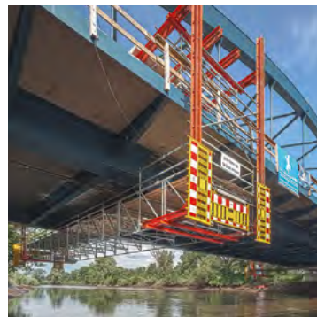
The manually portable scaffolding with its 20 m span is based on the LGS system and serves as a working platform for implementing corrosion protection measures.
