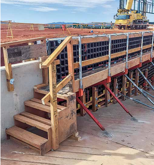
Using the DUO system resulted in a considerable increase in efficiency on the construction site.
