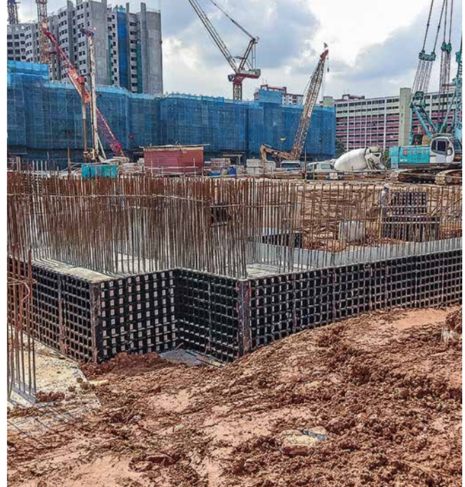
The DUO panels were ideal for forming small-scale concrete components with low surface requirements.
