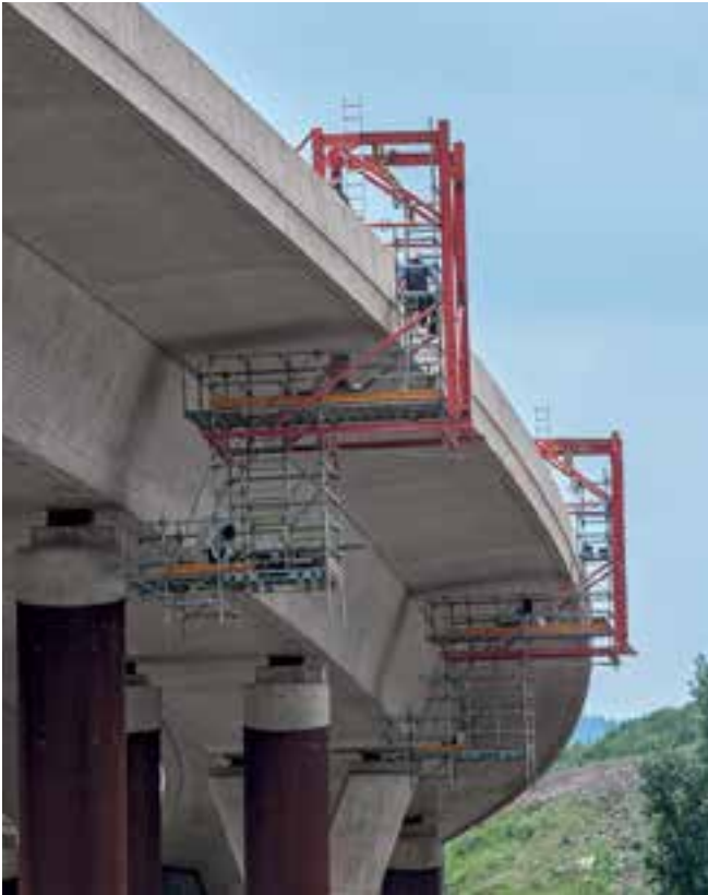
Two mobile PERI Suspended Scaffolds provided optimal access to the underside of a motorway bridge.
