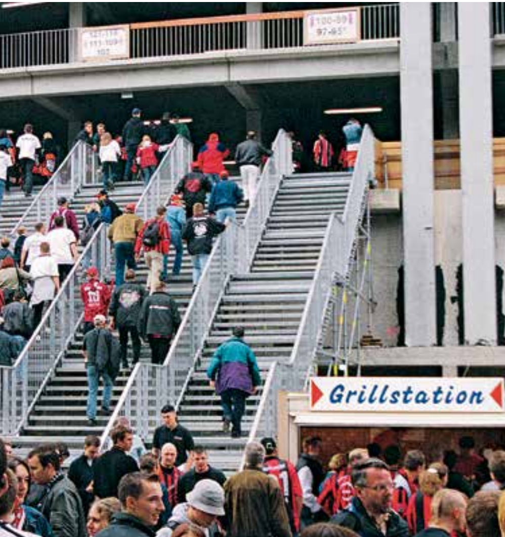
Bank of continuous staircases for the refurbishment of a football stadium. This bank of continuous staircases was needed for the football matches at weekends and was moved by crane to a storage area during the week to allow construction work to continue.
