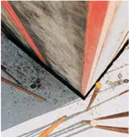
Clearly visible is the striking clearance of approx. 3 cm wide. The Shaft Panel itself remains close to the concrete thus allowing better guidance.
