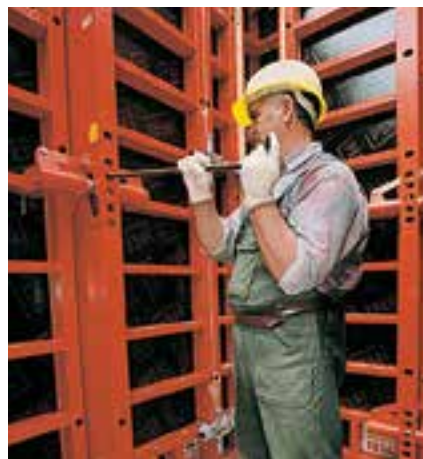
When striking, the crane slings are attached to all four Shaft Panels and the formwork panel is brought into the striking position by means of levering.
