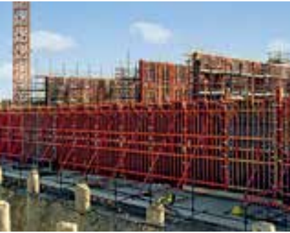
Kurnell Desalination Plant, Sydney, Australia
