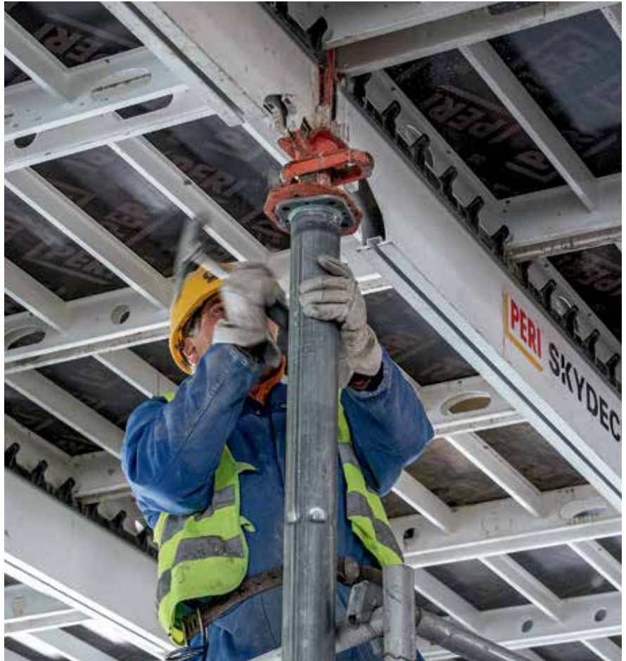
Easy and simple early striking: the formwork is lowered by 6 cm with just one blow of the hammer. After lowering the dropheads, the central panel is removed first followed by the neighbouring panels.
