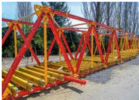
In order to ensure accessibility, the horizontal bracing is mounted on the outside of the pedestrian bridge by means of a simple, clever solution.
