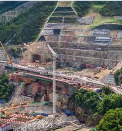
The Board of Management of the Chinese Permanent Cemeteries (BMCP) Footbridge, New Territories, Hong Kong
