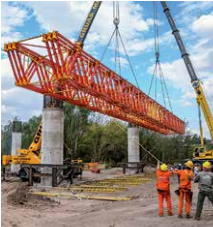
The lightweight towers and girder packages do not have to be split into multiple units for lifting purposes.
